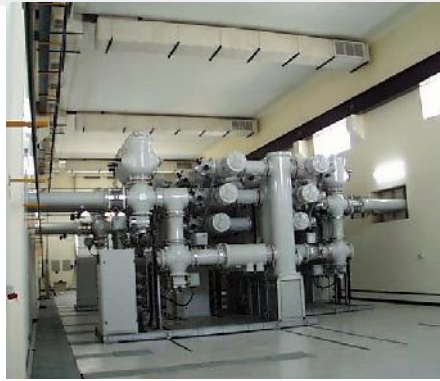
A Gas Insulated Substation (GIS), delivered by Siemens T&D to Sharjah in the United Arab Emirates
