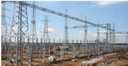
A typical regular high voltage substation
